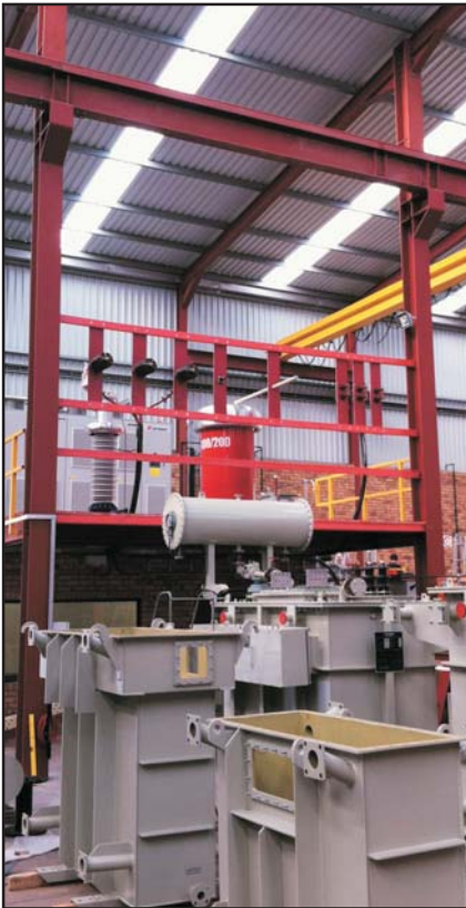
Saftronics Transformers. Test Laboratory with test a capacity up to 20MVA 132kV.
