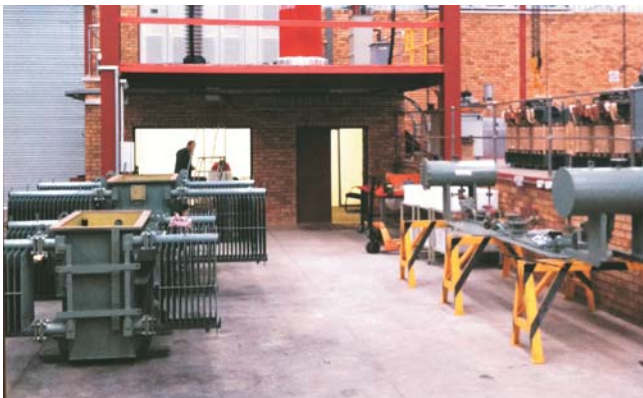
Transformers ready for Tanking.
